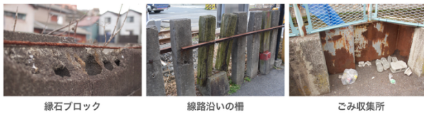
Fig.1 Deterioration of Concrete in Urban Areas
